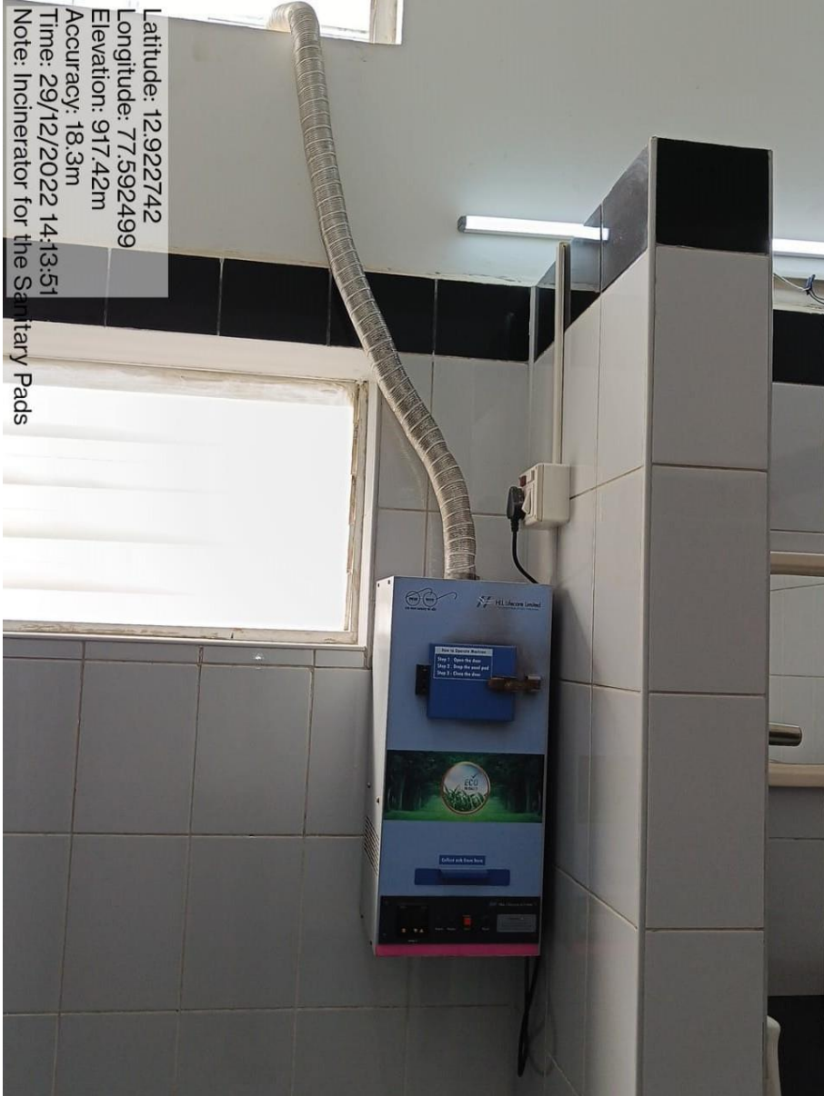
Installed Sanitary Pad Incinerator
