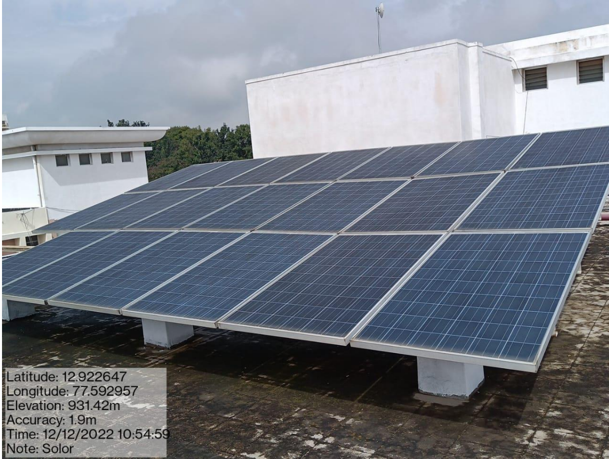
Solar Panel of 20KLD STP set up in the campus.
