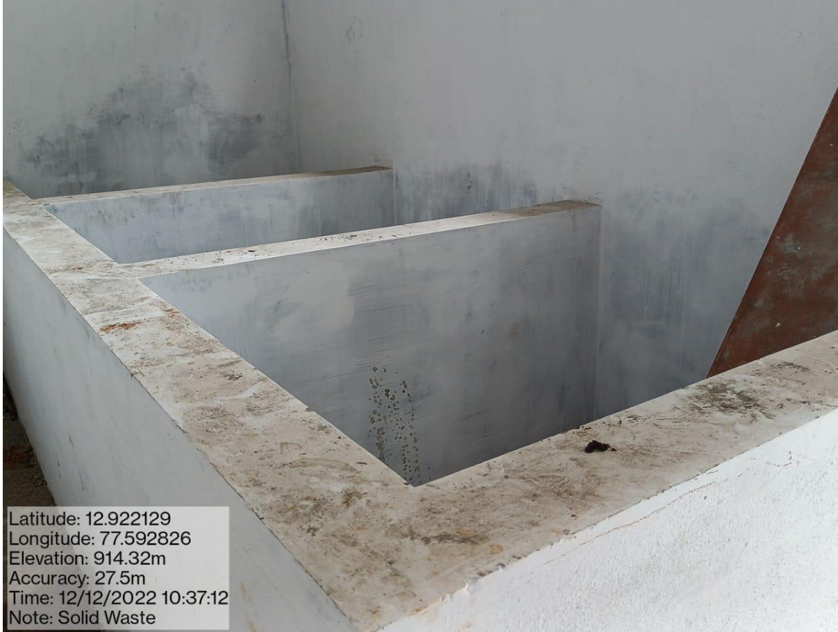
Solid Waste Collection pit in the Campus
