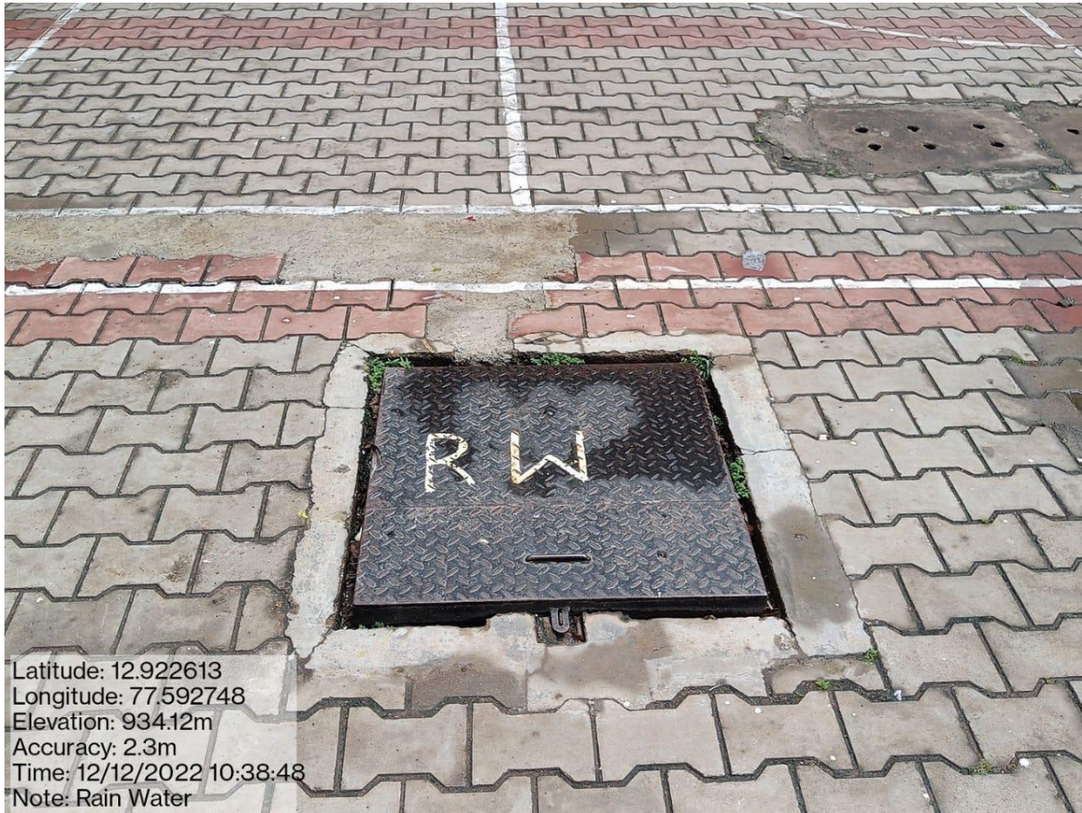
Rainwater Collection pit in the Campus
