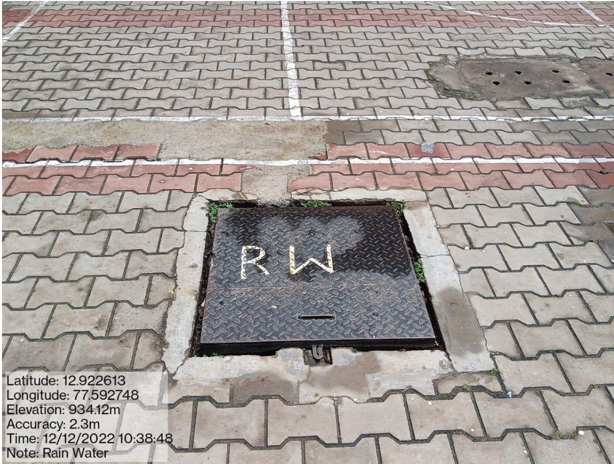
Rainwater Collection pit in the Campus
