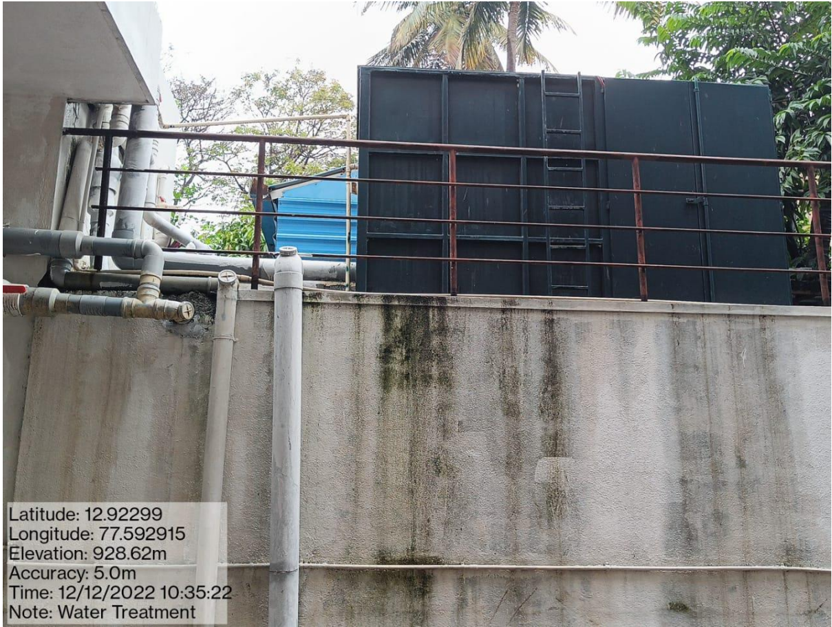
Water Treatment Plant in the Campus.
