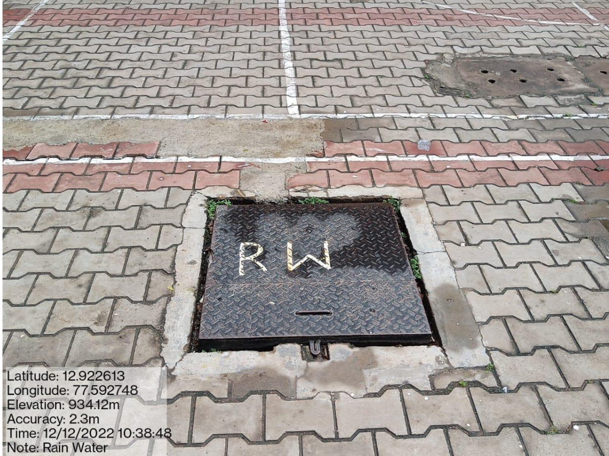
Rainwater Collection pit in the Campus
