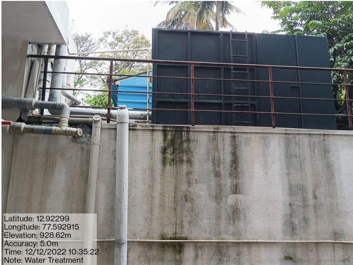
Water Treatment Plant in the Campus.
