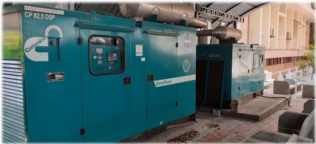
Diesel Generator (alternate source) during power cut
