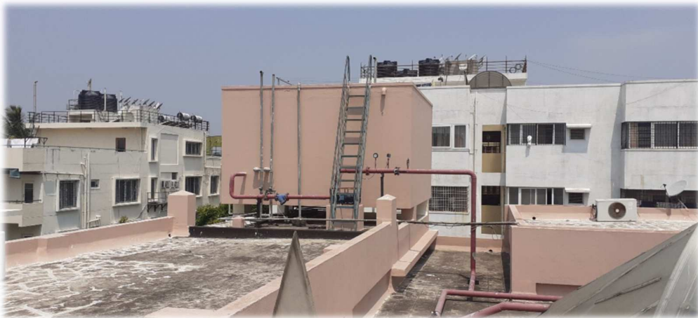
Overhead water storage tank
