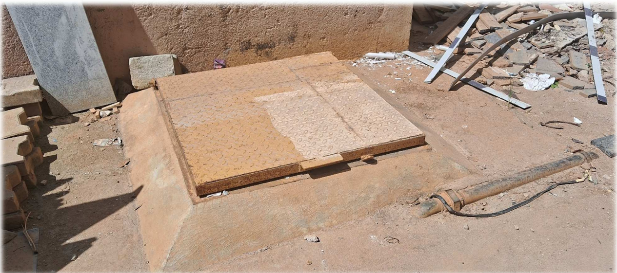
Water storage tank
