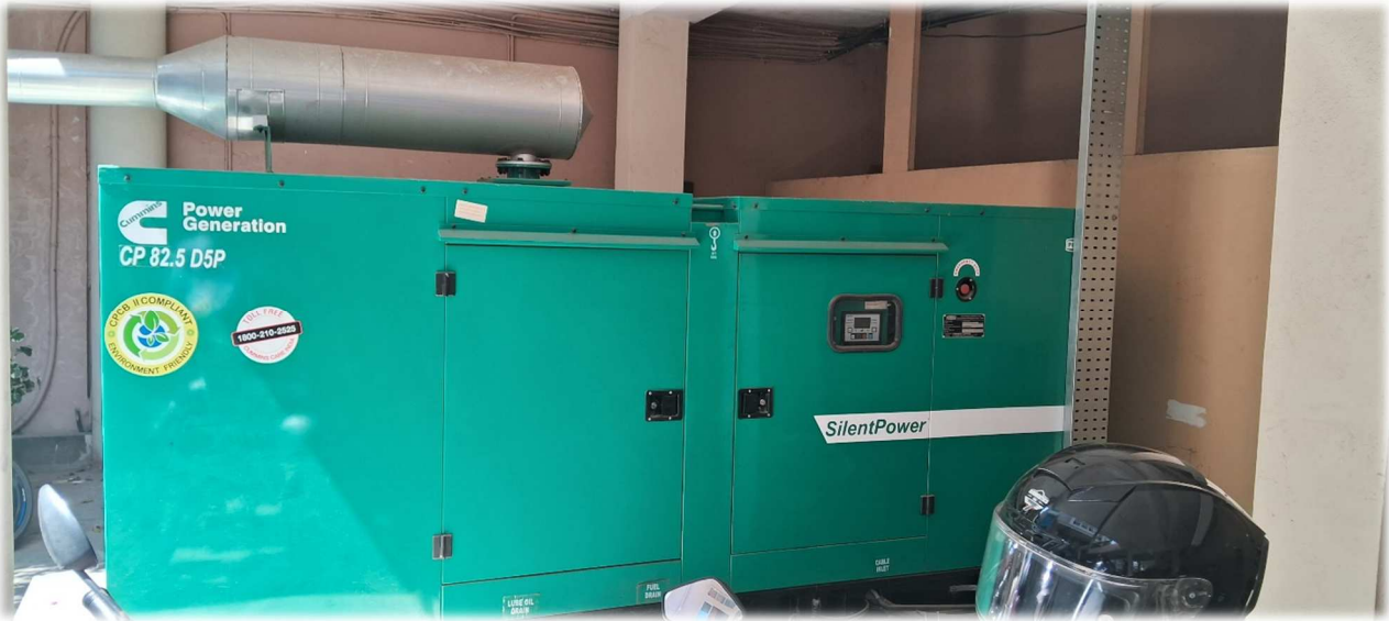
Diesel Generator (alternate source) during power cut
